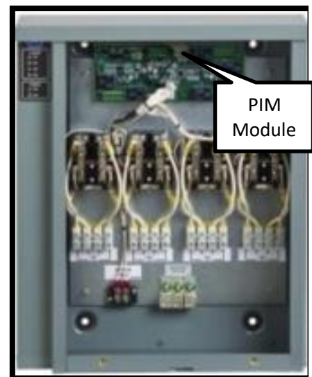
Kohler PIM Module installed
