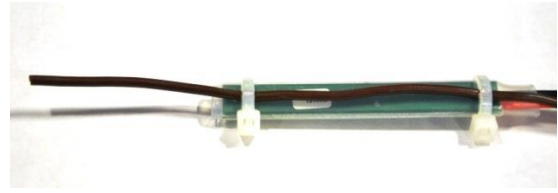
Rear View – AC Conductor on back of Detector
